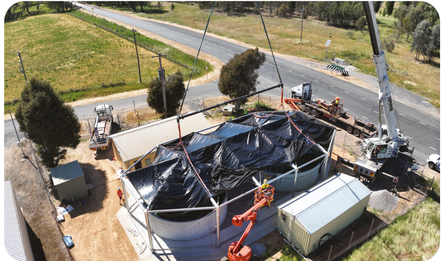
RAISING THE ROOF: Cranes install an aeration cover at Ralvona to protect treated water and maintain water quality.
