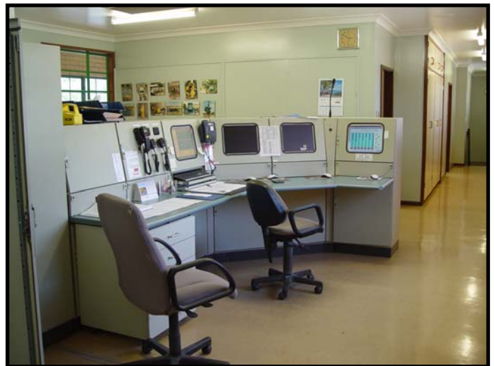
Control Room, Waterworks
